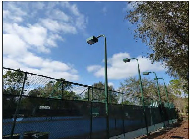
Tennis Court Lights
