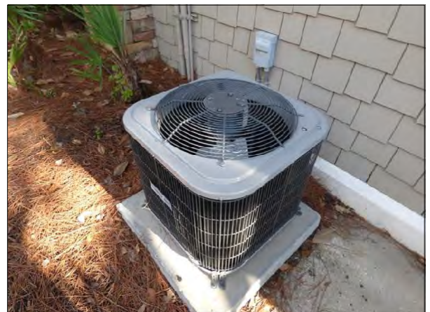
Ranger Station HVAC
