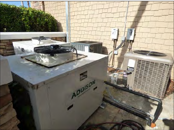
Fitness Center HVAC
